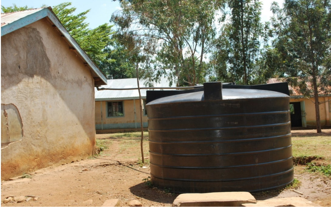
Figure 13: Rain water storage at Nduru-Kadero primary
